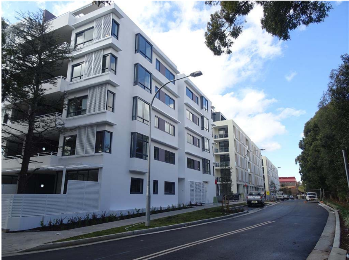
Figure 8: The southern edge of the site showing Building D, G and H nearing completion.
