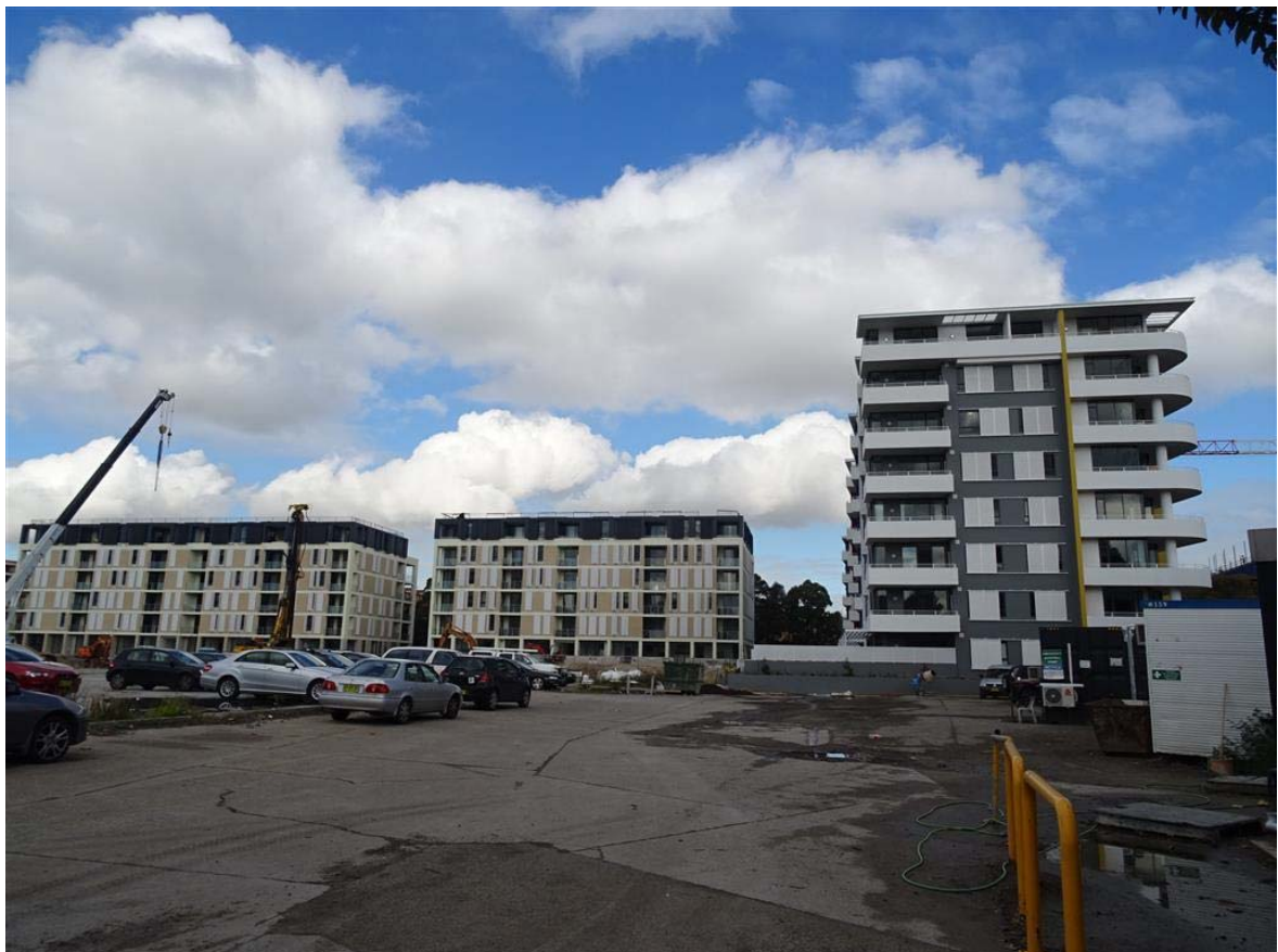
Figure 5: Looking south across the site showing Building H, G and D nearing completion.
